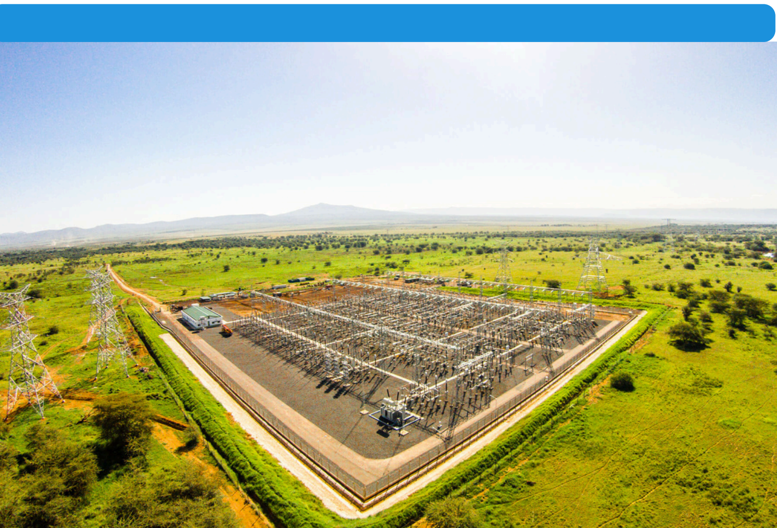
Image: KETRACO power station
